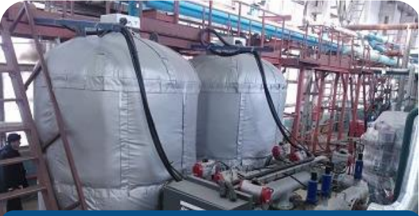
Leading Russian chemical company receiver thermal insulation
