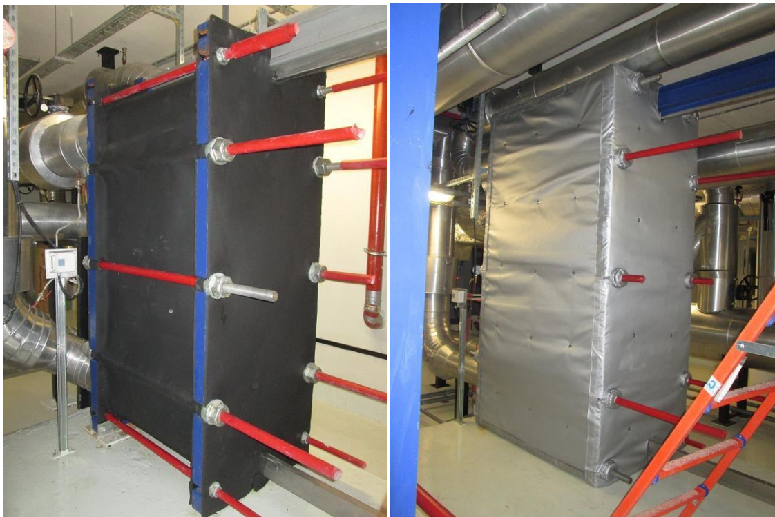
14. A-class business center. Thermal insulation of the heat exchanger in the air conditioning system.
