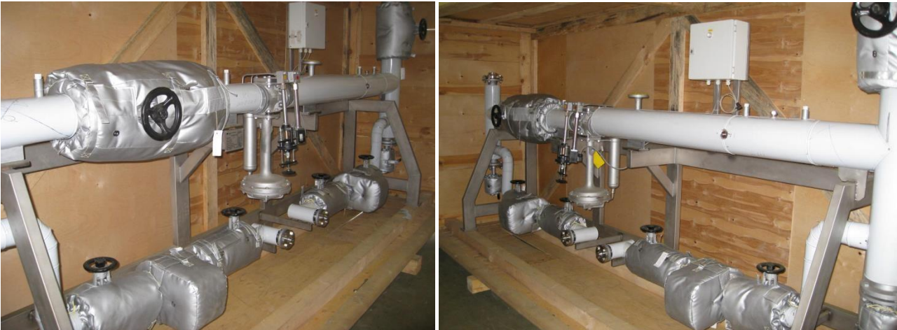
8. Engineering company. Thermal insulation of the reducing station.
