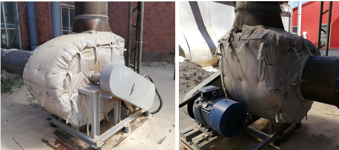
22. Furniture manufacturer. Soundproofing of an industrial fan.
