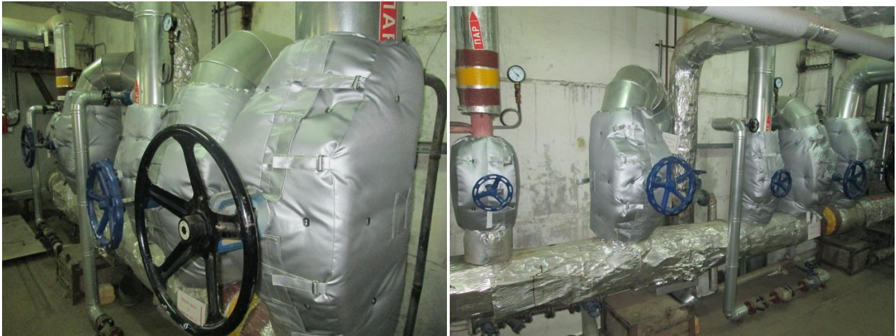
10. Leading American manufacturer of soft drinks. Thermal insulation of the boiler room.
