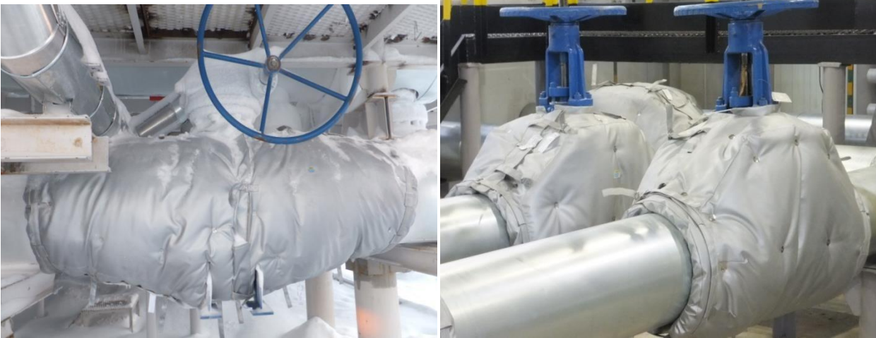
18. Russian oil and gas company in N. Urengoy. Thermal insulation of gas pipelines.
