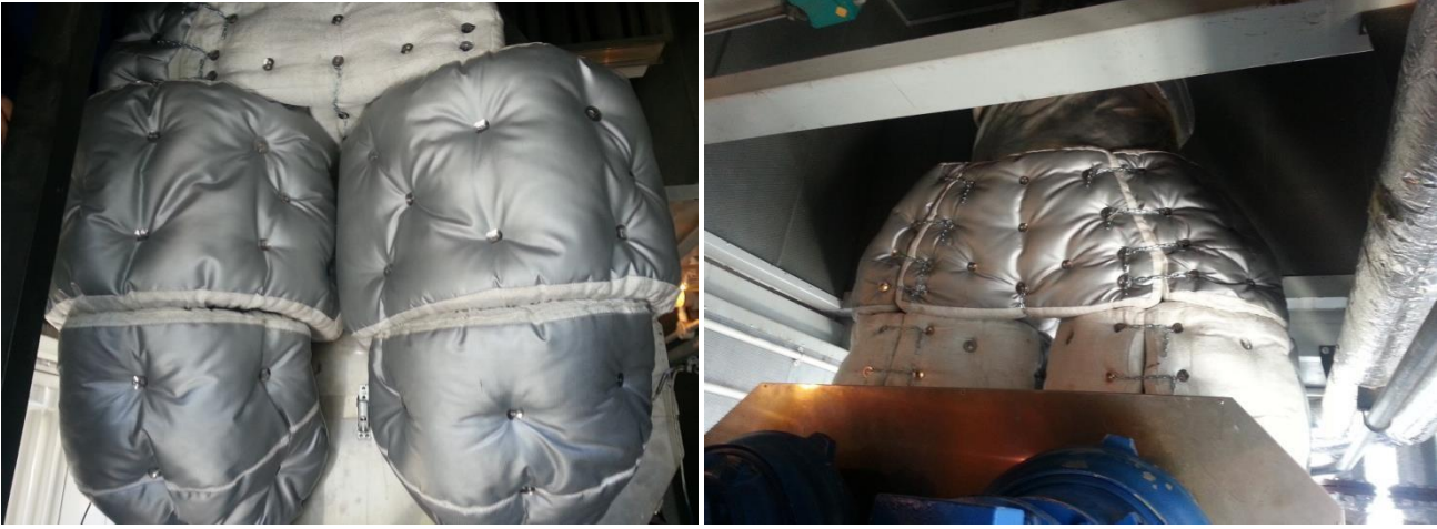
12. Power station. Thermal insulation of the exhaust system.
